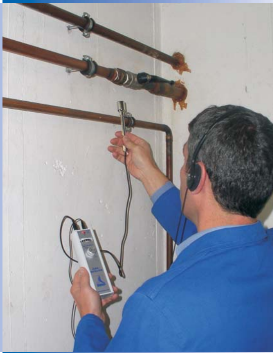
Acoustic signals lead directly and doubtlessly to the leak.
